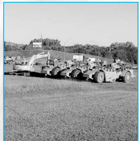
Ground breaking begins at the future site of Valley County Health System.
